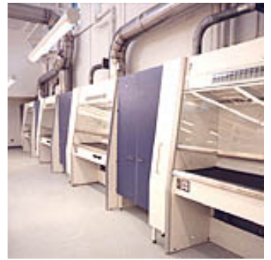
Fume hoods with ventilated storage cabinets.
